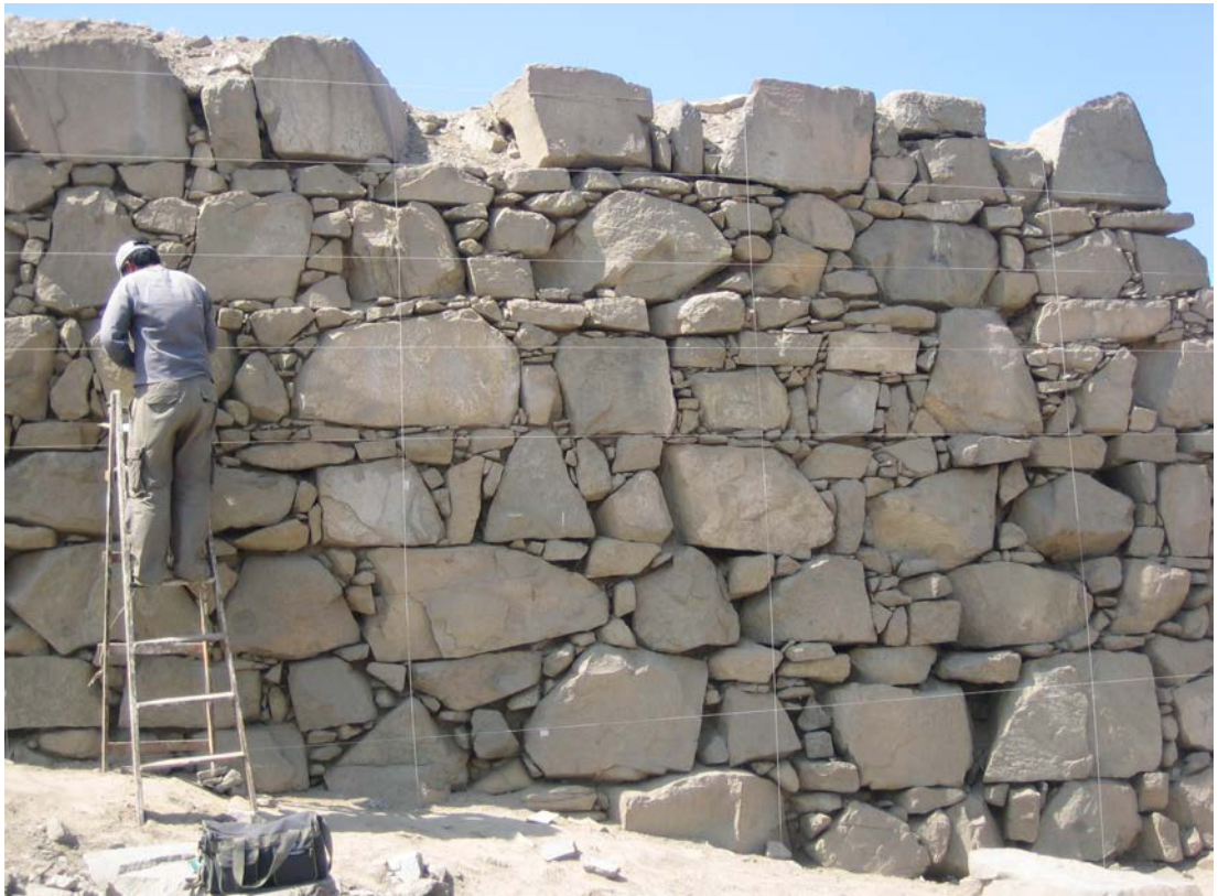
Figura 6. Detalle del muro norte de la EA 1. Detail of the North wall of EA 1.
